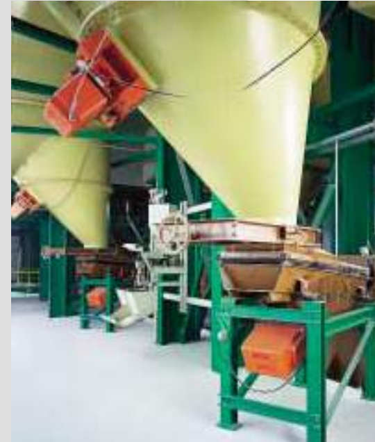
Continuous charging of ingredients for glass manufacture with feeding into the melting end takes place with finely controlled conveyor troughs with maintenance-free magnetic drives. Additional impact vibrators on the bunker walls prevent the material from caking to the sides and from forming bridges
